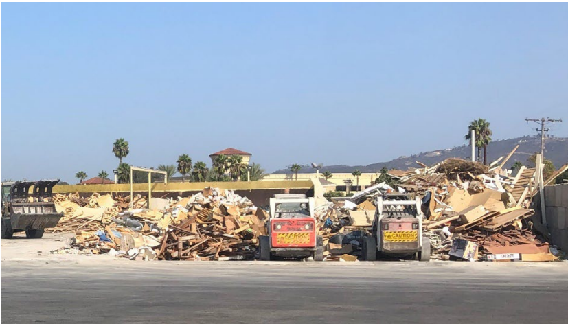
EDCO CDI Recycling Facility – San Marcos
